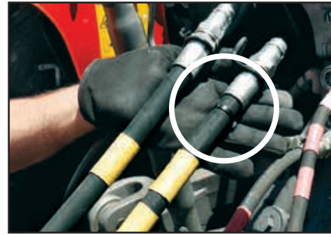
The Pressure Line hoses are identified by two coloured bands and a cable-tie.
