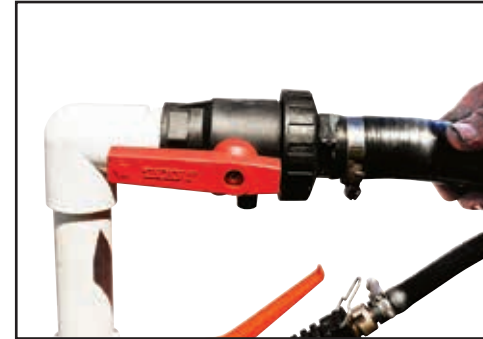
Open Probe valve to transfer mixture to spray tank.
