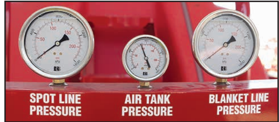
Pressure Gauges : Spot line, Air Tank & Blanket line
