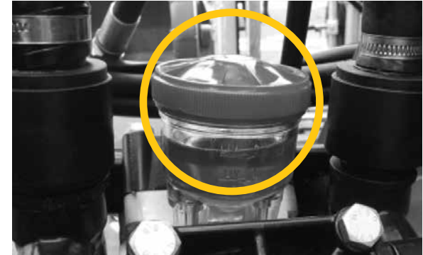
Check pump oil level
