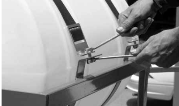
Regularly check that tank straps are tight
