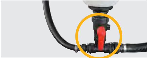
Open the Transfer valve to transfer the rinse mixture
