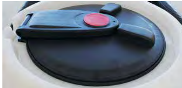
Main tank inspection lid closed & locked
