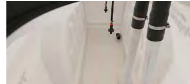
Visually check both tank agitators are working
