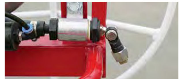
Check Fenceline nozzles are working correctly
