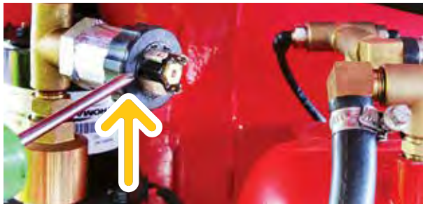
Adjust the level switch (hysteresis) set at 70 psi via the side hole on the valve [shown at end of screwdriver]
