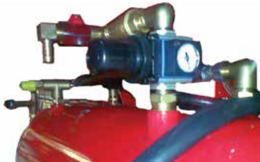
ARDS pressure control and drain valve
