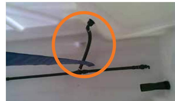
Sparge tube fitted in main tank
