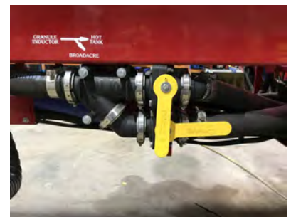
GRANULE INDUCTOR DIVERSION VALVES
