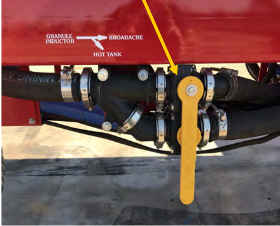
HOT TANK / BROADACRE TANK DIVERSION VALVES
