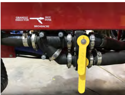
GRANULE INDUCTOR DIVERSION VALVES
