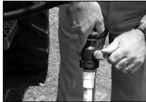
(h) Close the chemical probe valve.
