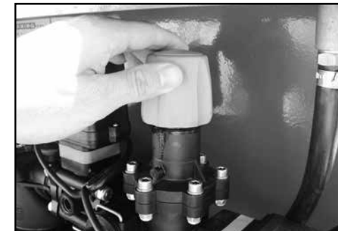
Adjust the manual pressure relief valve.
