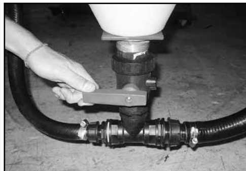
(g) Close transfer valve at the base of the hopper.
