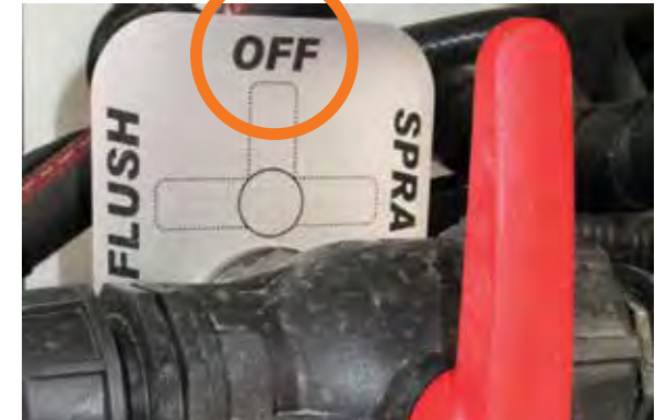
The pump suction valve CLOSED to the main tank
