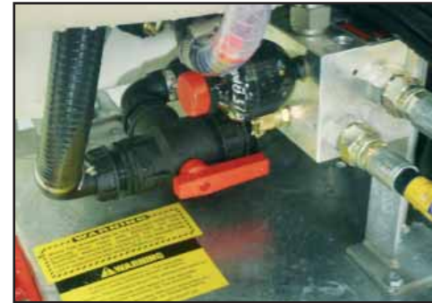
The pump suction valve OPEN to the main spray tank.
