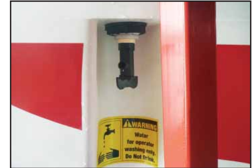
Fresh water tap for personal safety.
