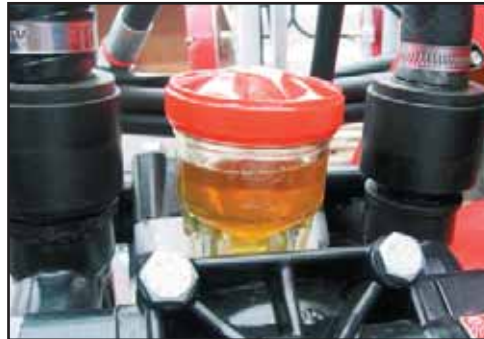
Check pump oil level.
