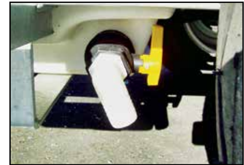
Tank drain valve CLOSED.
