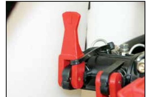
Liquid supply to heat exchanger with tap cable-tied in ON position.
