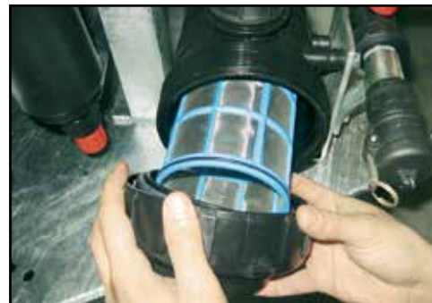
Check suction filter is clean.
