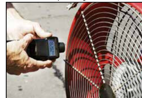
Check fan speed using an RPM meter.
