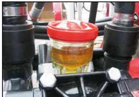
Check pump oil level.
