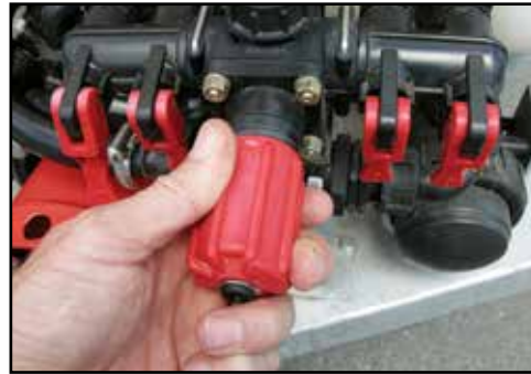
Adjust PRV for Pressure Control.
