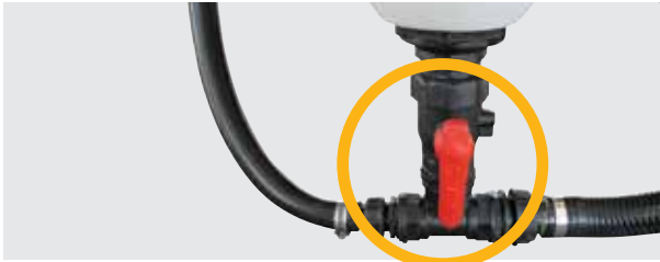
Open the Transfer valve to transfer the rinse mixture
