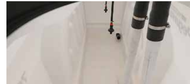
Visually check both tank agitators are working
