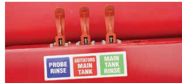
Open the "Probe Rinse", "Agitators Main Tank" & "Main Tank Rinse" valves
