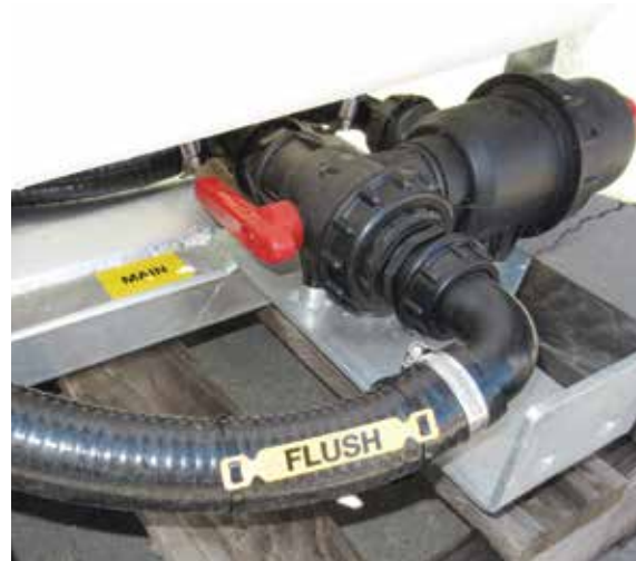
The pump suction valve CLOSED to the main tank
